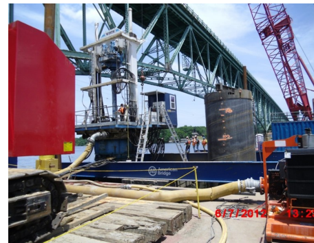
Fig 3b: Reverse Circulation Drill Rig Foundation drilled the rock sockets with an RCD rig. The rig was mounted to the top of the permanent casing as shown in Figures 3a and 3b and the excavation was advance using a full-face cutter assembly as shown in Figure 4.
