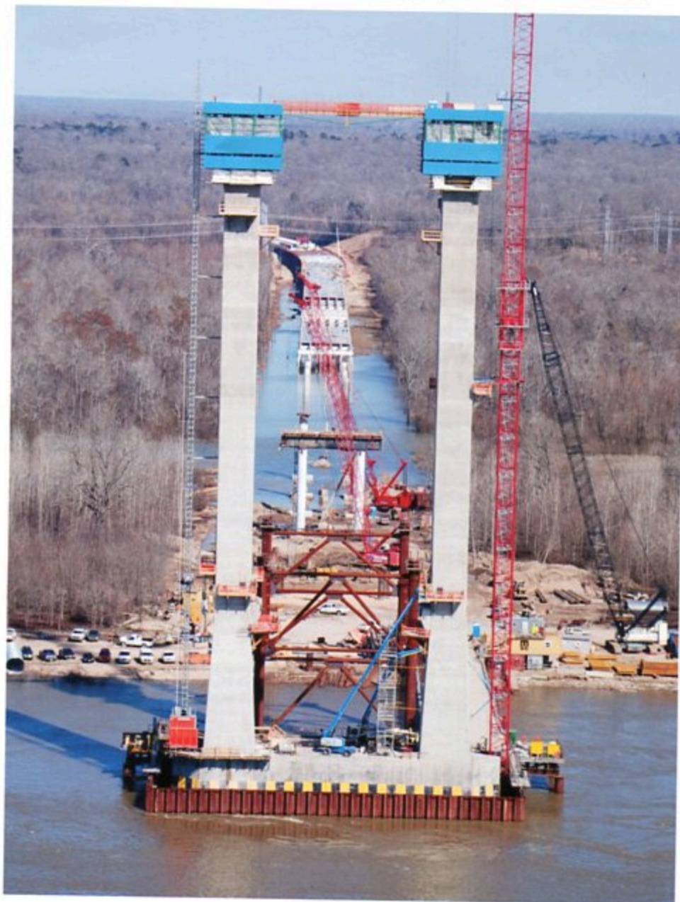
Below: West pylon construction in foreground with high-level approach construction looking west
