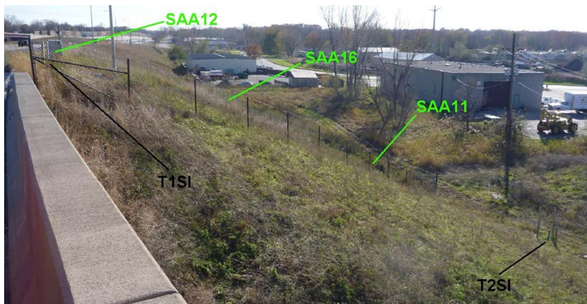
Figure 3. The embankment fill is shown looking southwest from the adjacent bridge. T1SI and T2SI are borings with slotted casing for manual traversing probe inclinometer use. Installations SAA11, SAA12, and SAA 16 are outfitted with automated ShapeAccelArray sensors.
