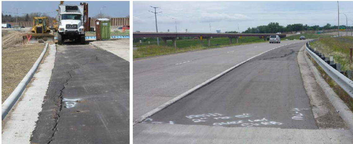
Figure 2. Distress cracks in the bituminous shoulder were seen during construction shortly after the bituminous shoulder was placed (left) in April 2008. New distress is seen (right) in June 2010.
