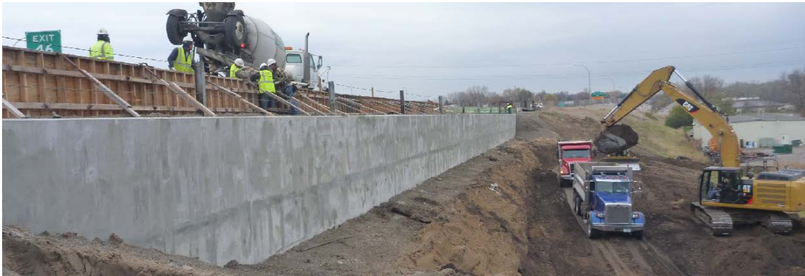
Figure 10. A ten inch thick permanent structural concrete wall was cast in front of the piles.
