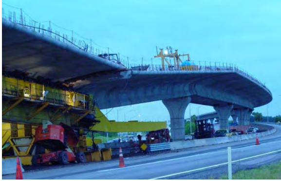
Figure 4. Pier 97 Failure During REL work.
