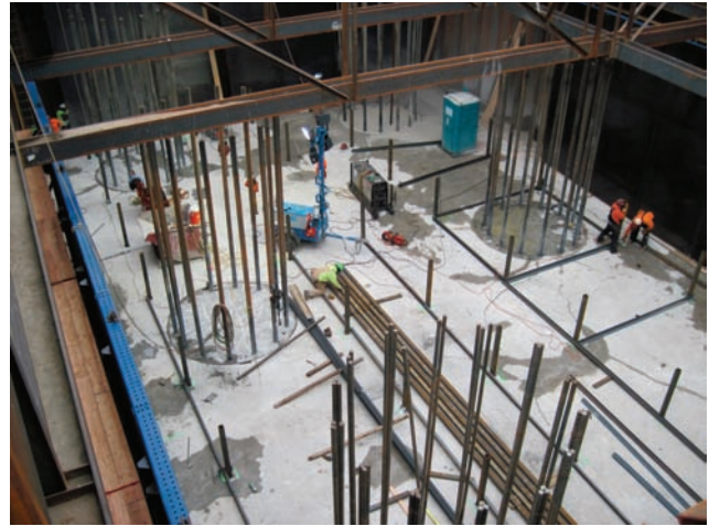
[FIG. 16] Construction of the Pylon Foundation within Coffercell at Top of Seal
