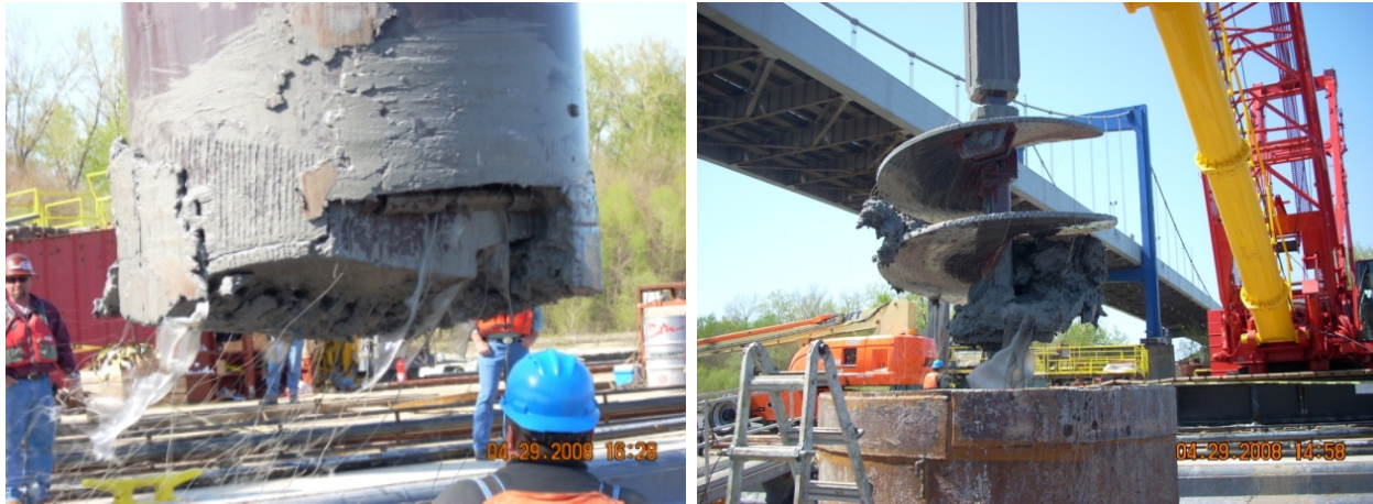
Figure 8: 6-ft diameter drilling bucket and auger used for excavation of test shaft.
