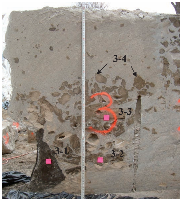
[FIG. 9] Soil inclusions and vertical hole from post-construction coring in triple fluid jet grout column #3.
