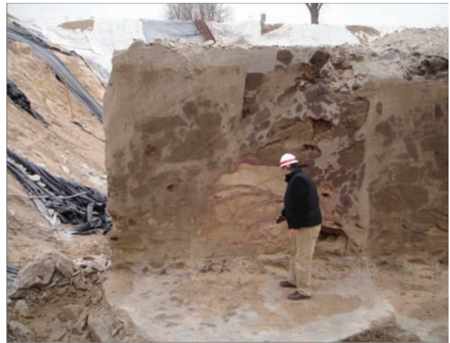
[FIG. 7] Close up of sectioned triple fluid jet grout columns 10-11-12 (10 ft diameter)
