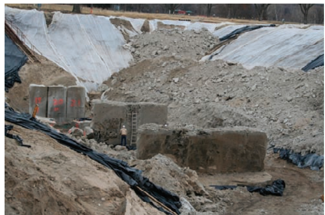
[FIG. 6] Sectioned double and triple fluid jet grout and soil mix column using a diamond wire saw.
