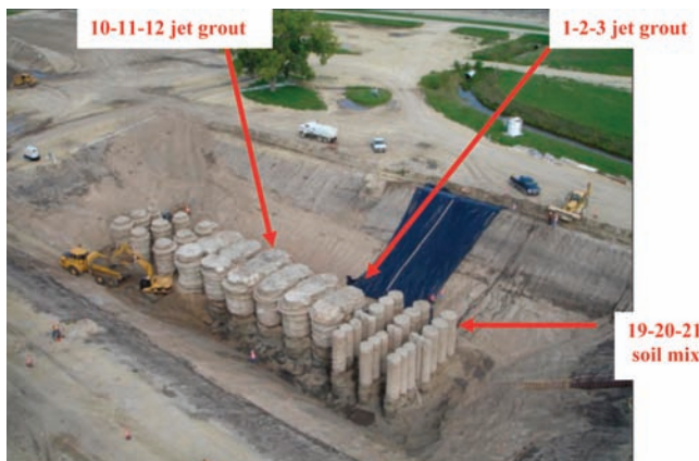
[FIG. 5] Jet grout and soil mix columns during excavation and columns to be sectioned.
