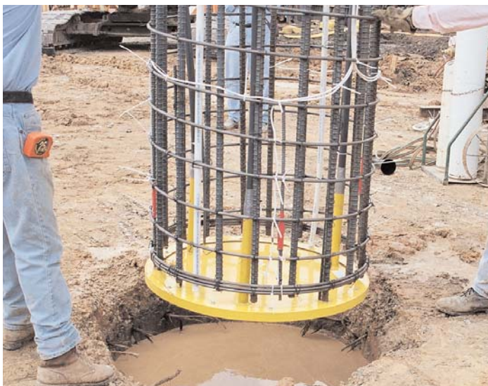
Grout Distribution System on Shaft Base
