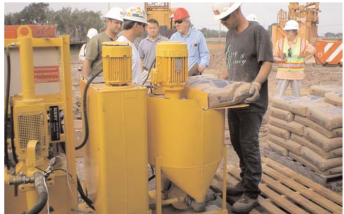
High Pressure Grout Plant
